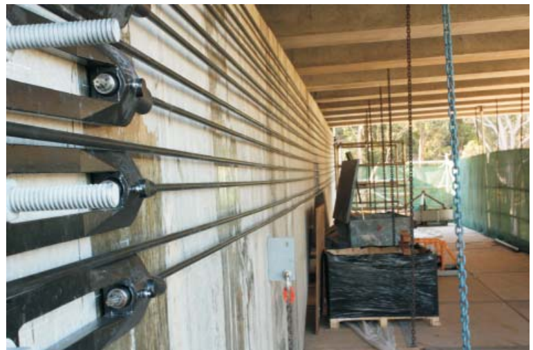
Pier headstock strengthening, Sydney, Australia
