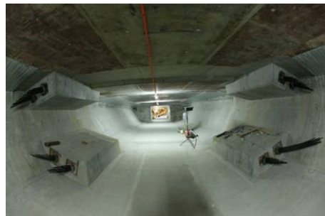
Fig. 10 . Blisters inside the box girder. Dead end anchors are visible with strands uncut
