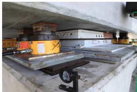
Fig. 22. Jacking of the deck and shifting of pots to their permanent position
